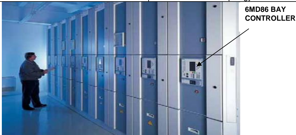
Gambar : Protection Relay 6MD86 dipasang di switchgear dan panel.
