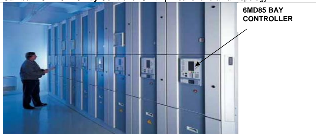
Gambar : Protection Relay 6MD85 dipasang di switchgear dan panel.
